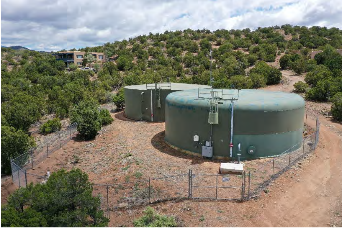
Figure D5. Tanks1- 1A
