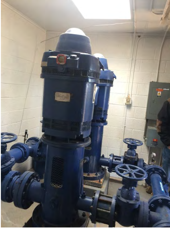
Figure D11. Well 9 Booster Pumps
