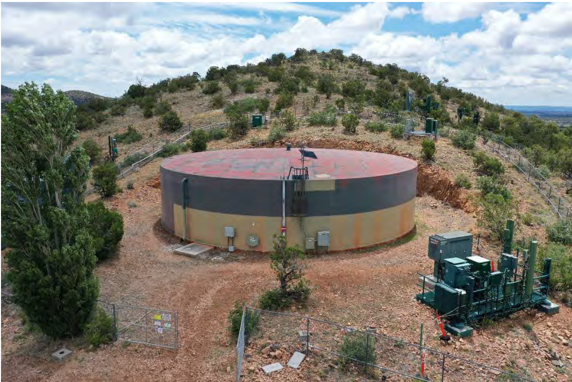
Figure D6. Tank 3
