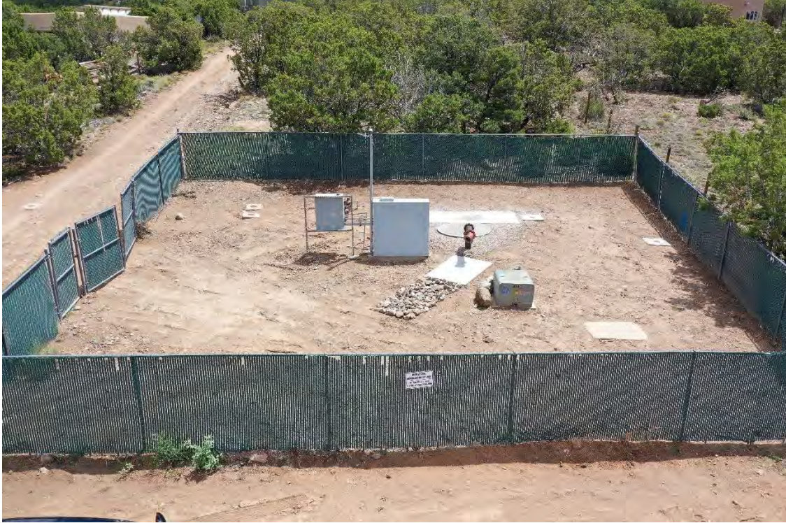
Figure D3. Tank 1 Booster Pump Station
