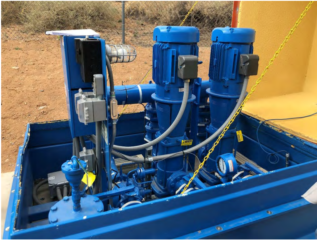
Figure D4. Tank 4 Booster Pump Station
