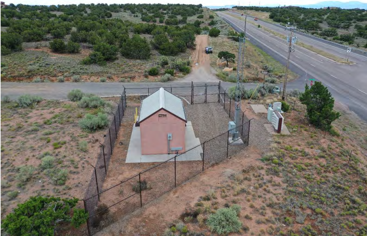
Figure D1. Old Ranch Road Booster Pump Station
