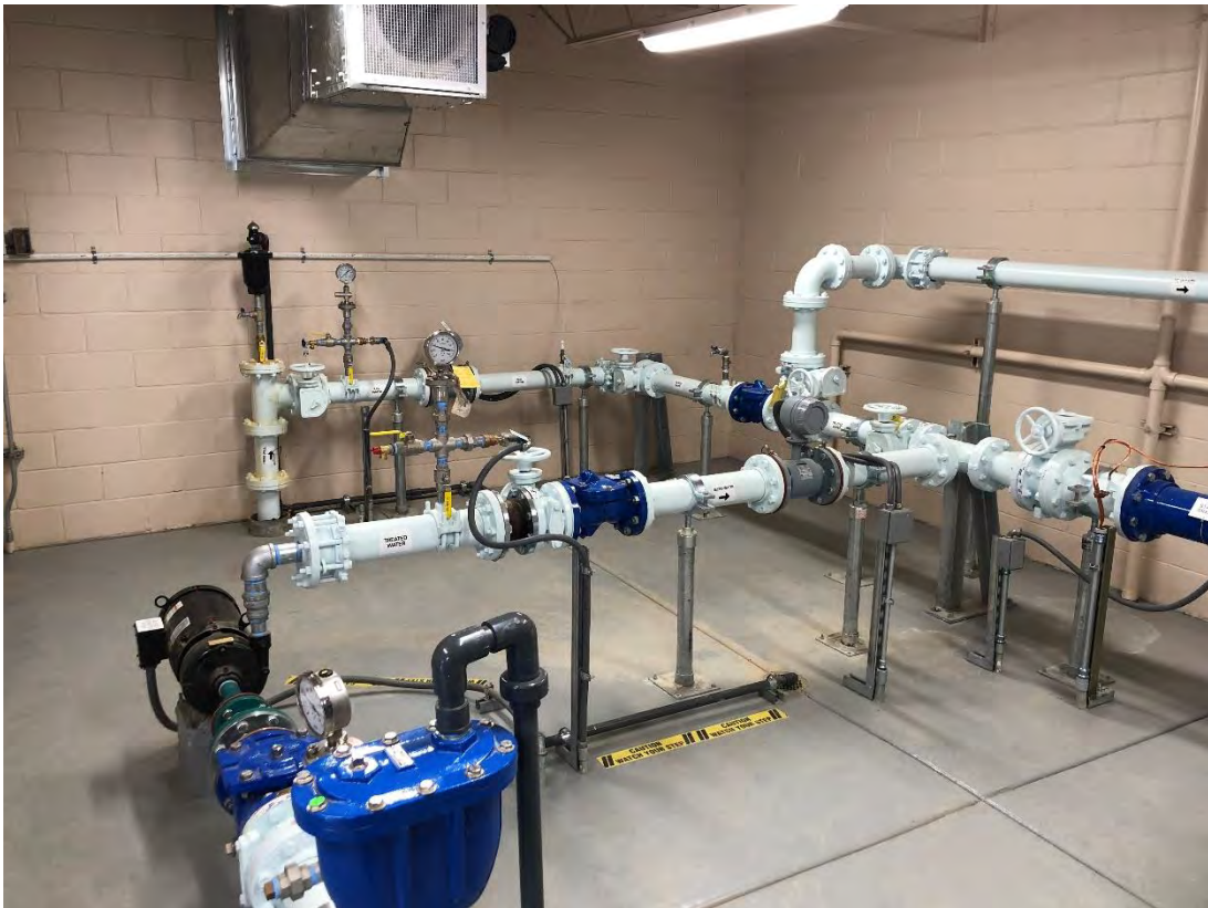
Figure D15. Well 19 Blend and Process Piping
